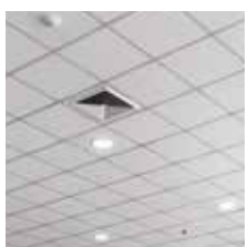
CEILING GRID FALSE CEILING
